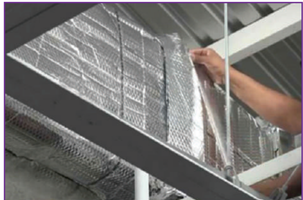
Ductwork Class 1 insulation with aluminium foil.
